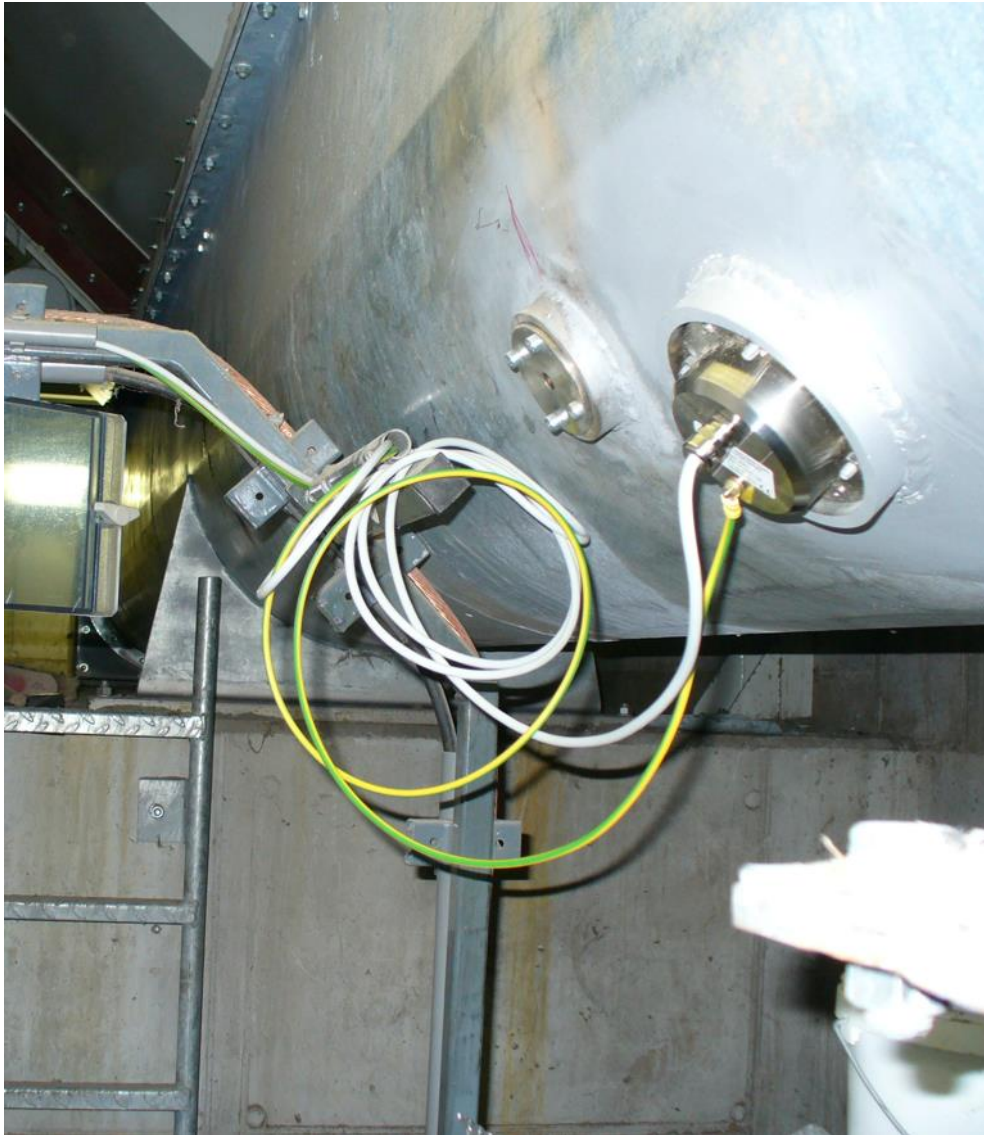
Measurement spot at the screw conveyor
