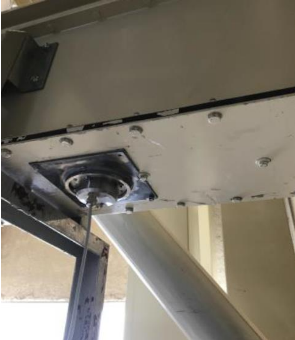
Sensor mounted at the bottom of a chain conveyor
