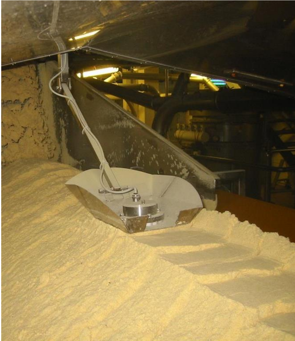
HUMY 3000 on the conditioning conveyor belt
