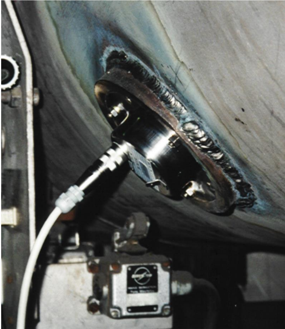
Measurement spot at the screw conveyor
