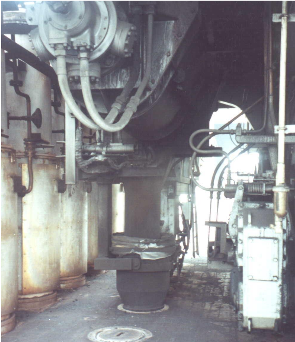
A Humy 3000 is installed in a hopper
