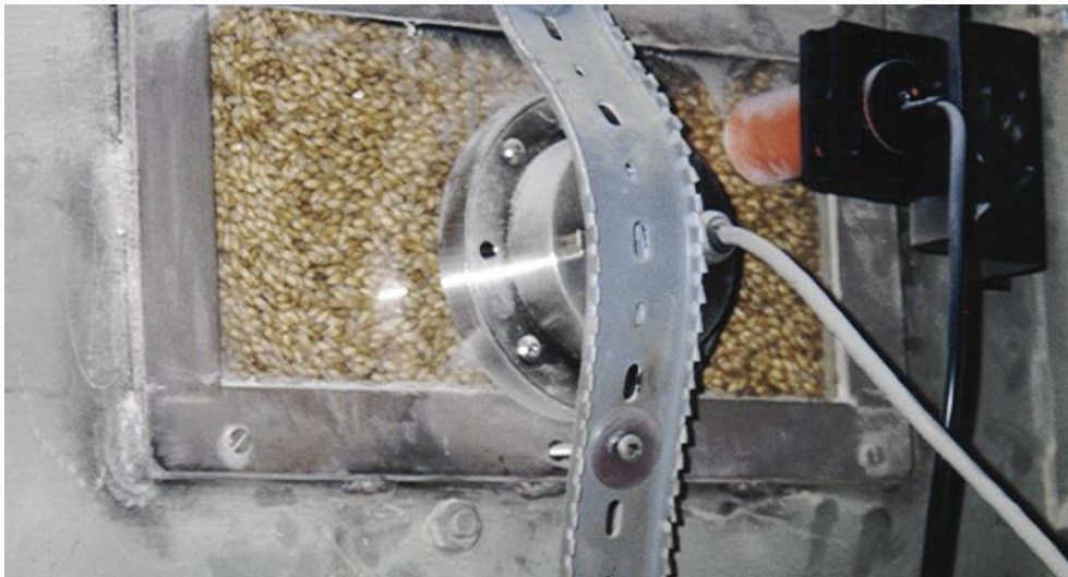
A sensor mounted on the closed chain conveyor in a malt factory
