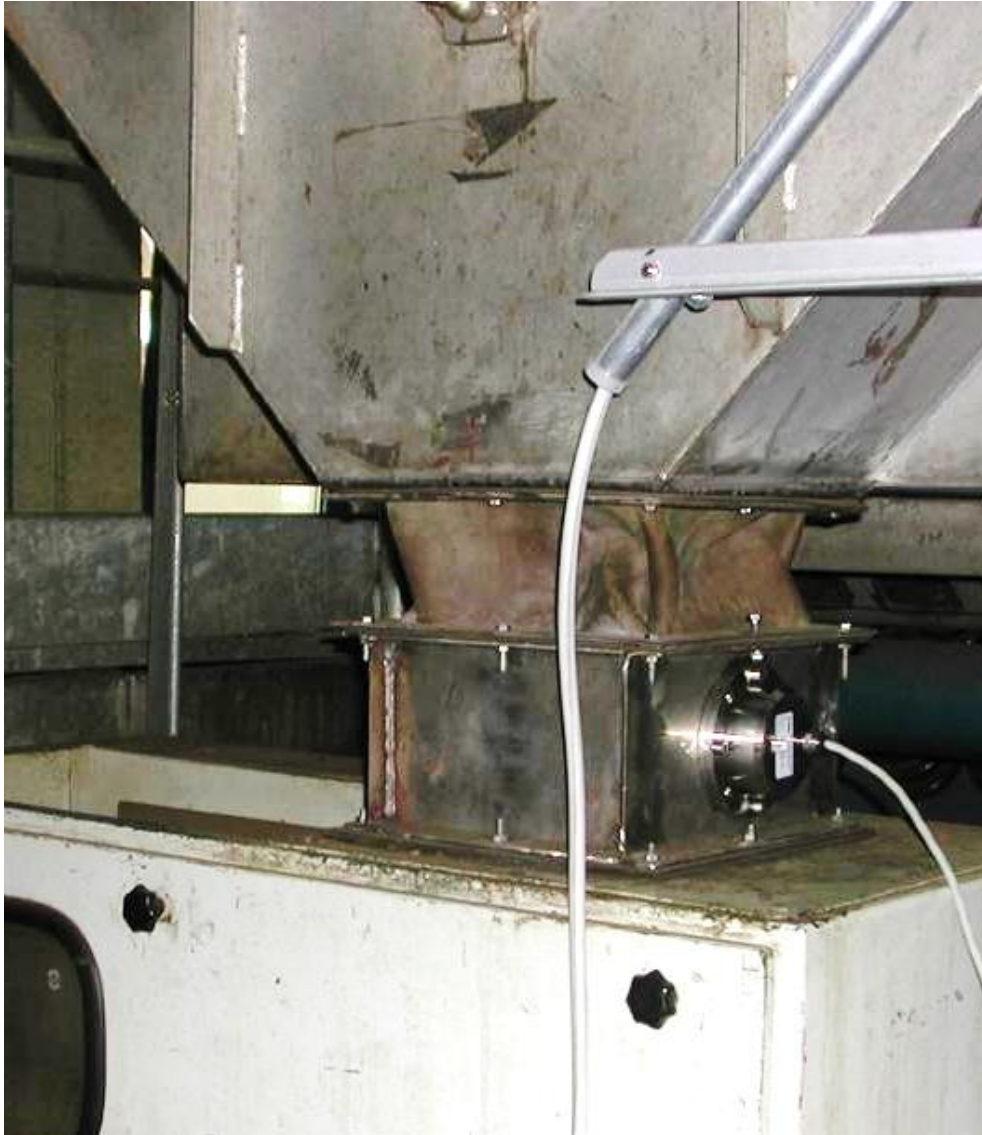
A Humy 3000 is installed between dryer and roastery
