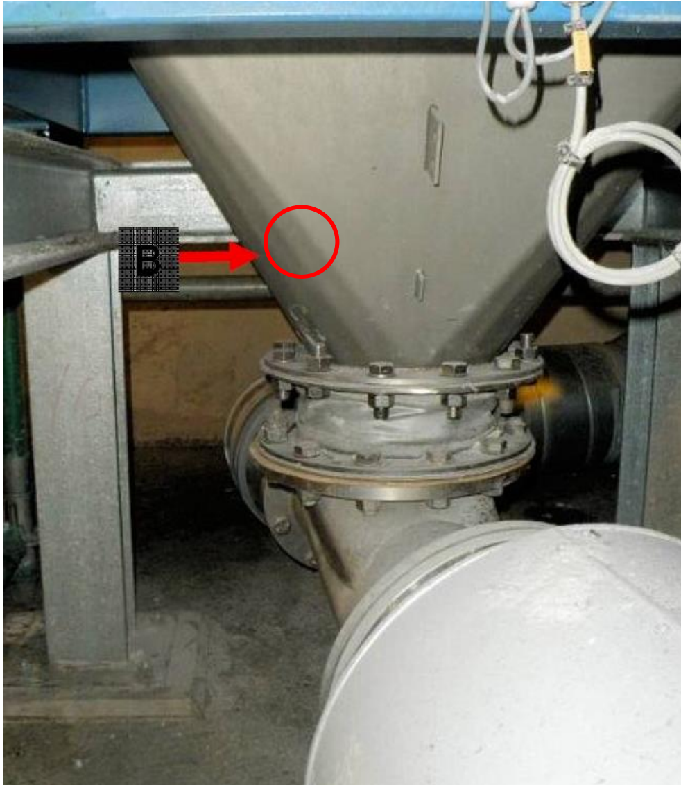
A Humy 3000 is installed at a hopper after the drying
